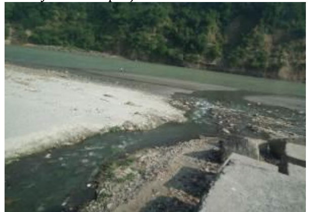
Raw Sewer flowing in Rain water drain and meeting with River Ganga (Existing condition)
