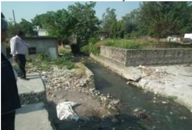
Raw sewer is flowing in natural rain water drain (Existing conditions)
